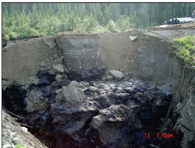
A massive road breach - ancient permafrost exposed
